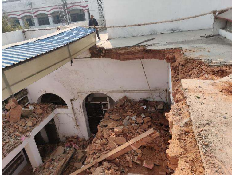
Image 8 Fallen Roof of the Main Hall
