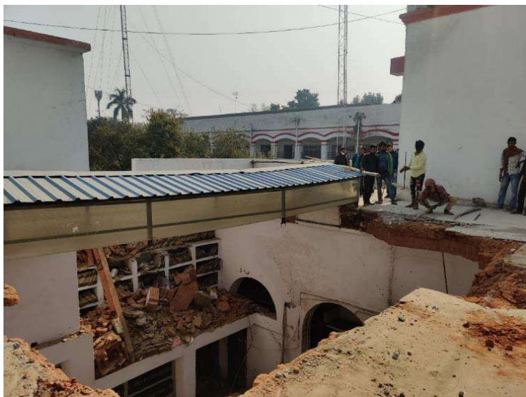
Image 9 View two of fallen roof structure
